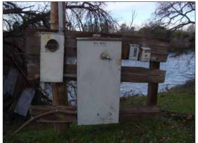
PHOTO 6: Electrical boxes associated with transformer along northwestern corner of Subject Property.
