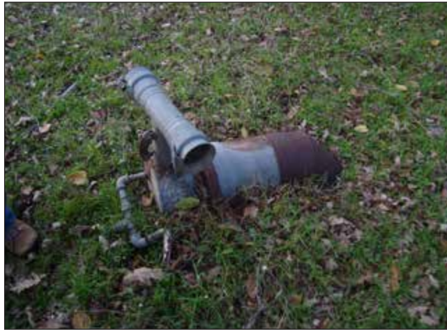
PHOTO 1: Portion of underground piping system visible in the northwest corner of the Subject Property.
