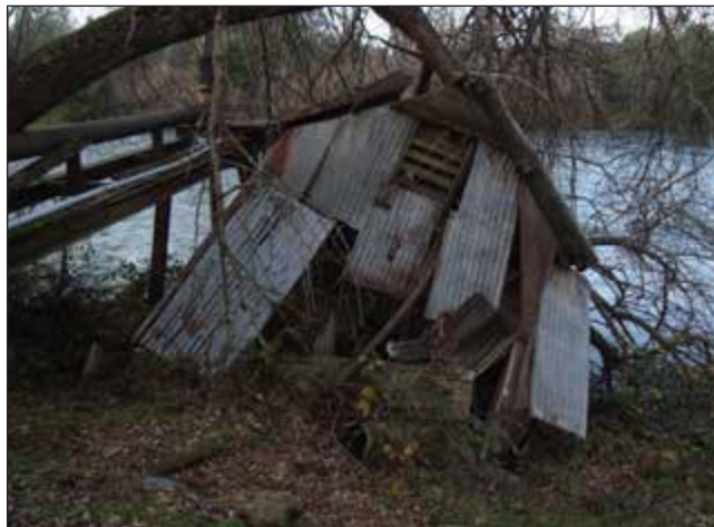
PHOTO 5: Rusty sheet metal structure collapsed onto bank of Sacramento River on northwestern corner of Subject Property.
