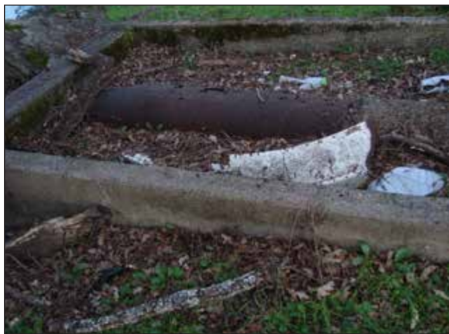
PHOTO 3: Rusty water pipe encased with concrete and scattered debris along the Sacramento River in the northwestern corner of the Subject Property.
