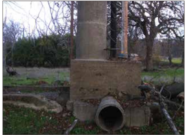
PHOTO 2: Concrete water distribution structure in the northwest corner of the Subject Property.
