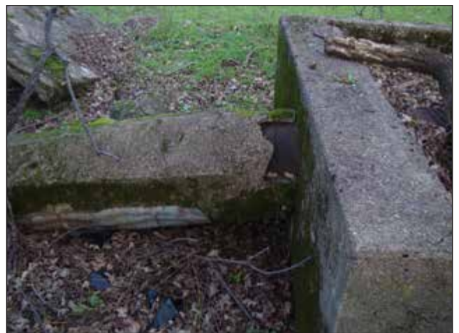
PHOTO 4: Rusty water pipe encased with concrete along the Sacramento River in the northwestern corner of the Subject Property.
